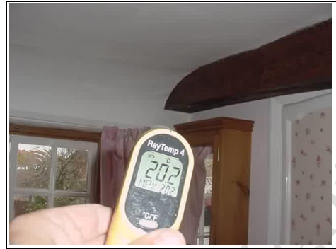
Slightly rounded ceiling in rear bedroom indicates the possibility of cold bridging
