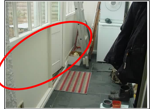
Base of rear lean to area with possible Asbestos
