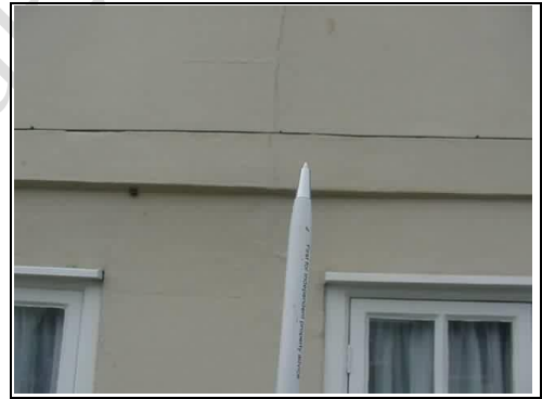
Cracking to render
