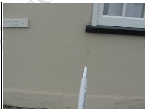
Cracking occurring to render
