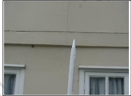
Cracking to render
