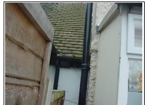
Unused soil and vent pipe to right of property
