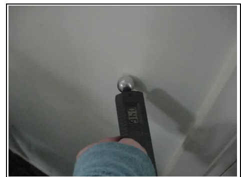
Damp meter reading indicating rising damp
