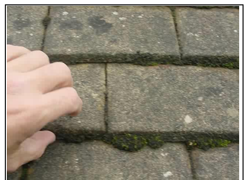
Moss gathering on roof tiles
