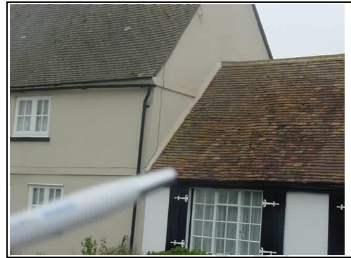
Poor quality roof detailing
