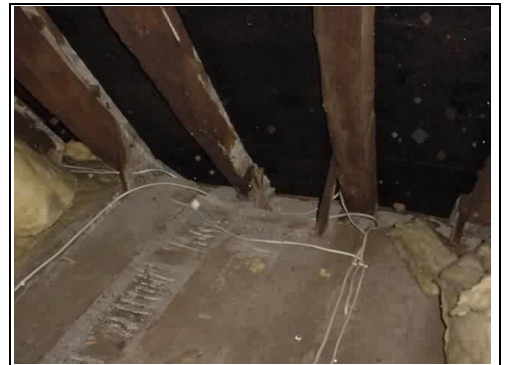
Wiring in the roof
