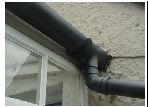
Awkward gutter and downpipe detail
