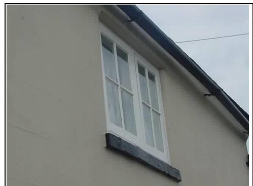
Render has cracking
