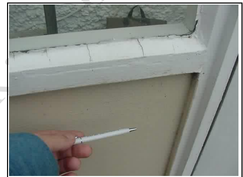
Possible asbestos to base
