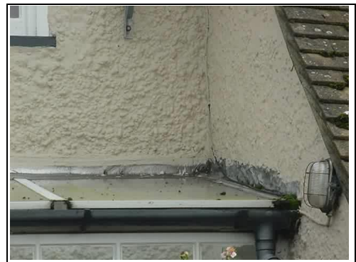
Poor detailing to rear low level roof
