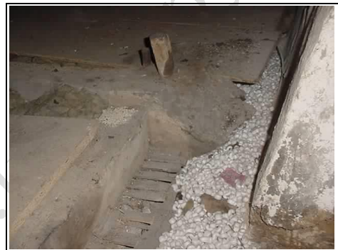
Spine beam not tied into frame within the roof
