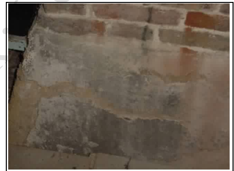
Damp plaster to chimney breast
