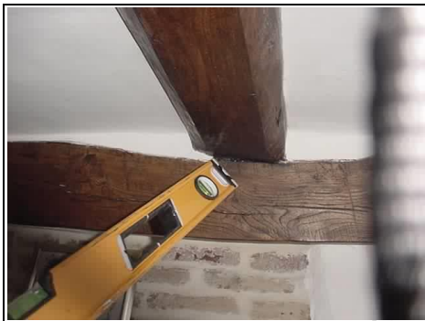
Beam does not look to be tied into the frame
