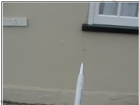
Cracking occurring to render
