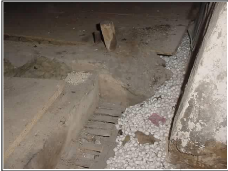
Spine beam that does not tie in
