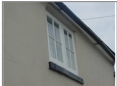
Render has cracking
