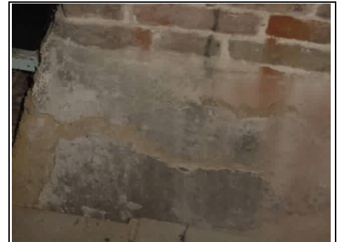
Dampness to chimney breast in roof
