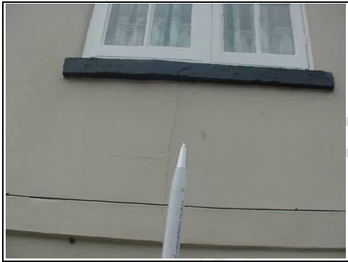
Cracks in render
