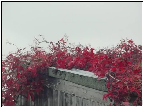
Overgrown plant on garage roof
