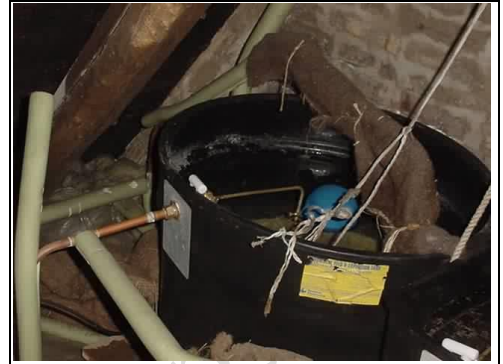
Un-insulated water tank
