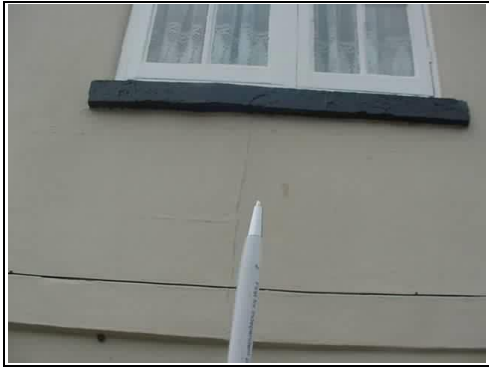
Cracks in render
