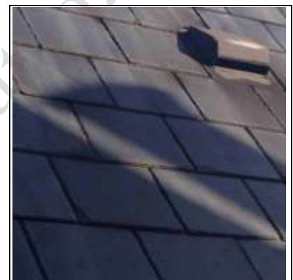
Vent on main/loft conversion roof
