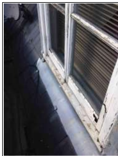
Timber window is deteriorating
