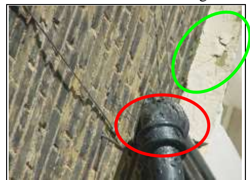
Cast iron pipe (red circle) and moulding (green circle) in need of redecoration
