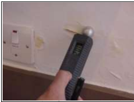
Dampness on fourth floor from box gutters above
