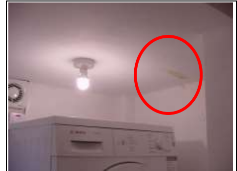
Staining on ceiling in utilities room on lower ground floor
