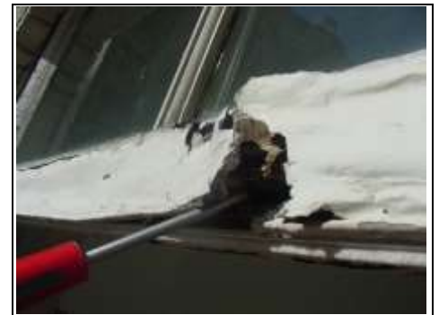
Window sills and ledges allow water to sit on them
