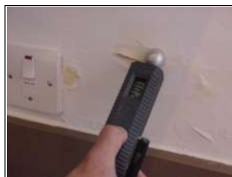
Dampness internally caused by box guttering to front wall
