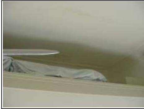
Staining in second floor bedroom from bathroom above
