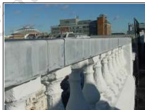
Lead capping to front balustrade
