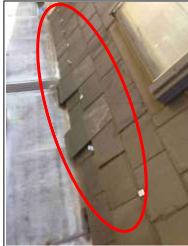
Left hand view of roof; far too many lead tingles and slates completely slipped
