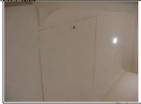
Loft hatch painted shut on lower ground floor
