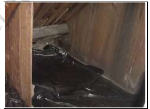
Dampness getting into roof on fifth floor
