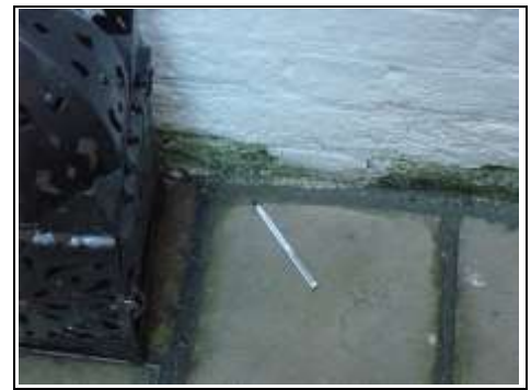
Painted brickwork to rear with areas of mould to the base
