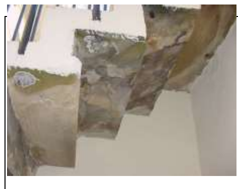
Underside of steps showing water getting through
