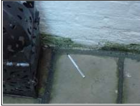
Tiled floor with areas of mould
