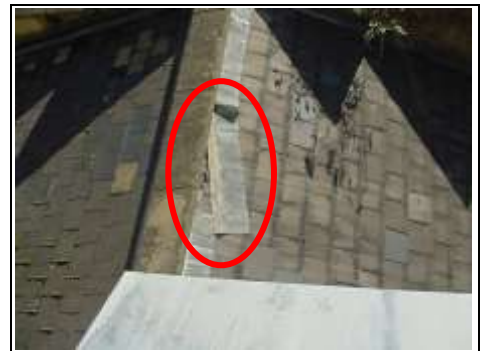
Lead flashing coming away on rear single pitched roof to your side
