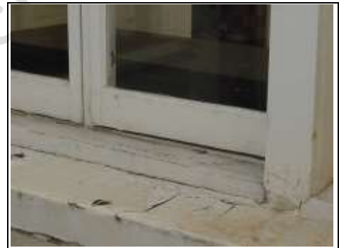
Windows generally need repair
