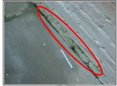
Mould around outside of walls in void area indicating
