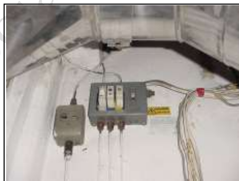
Electrics in boiler room
