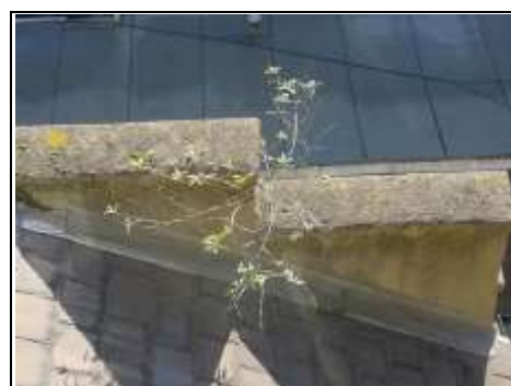
Plant growing out of parapet wall
