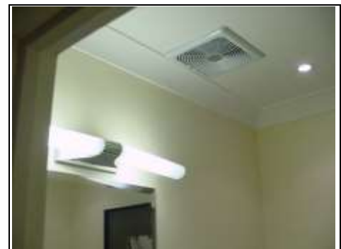
Extract fan on lower ground floor
