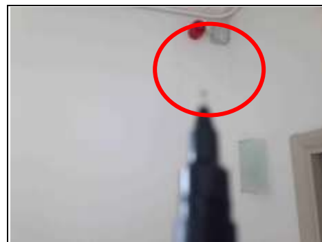
Crack in wall
