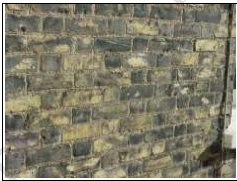
Rear brickwork where ad hoc repointing is needed
