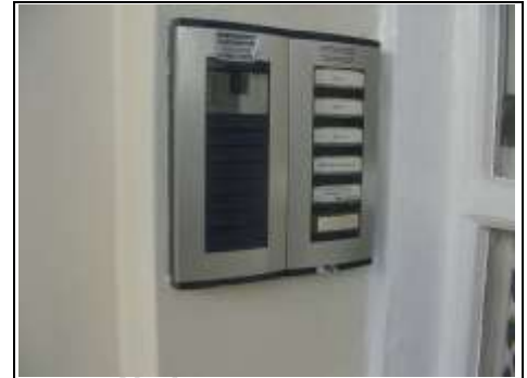
Door entry system
