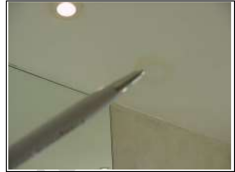
Staining in second floor bathroom from apartment above
