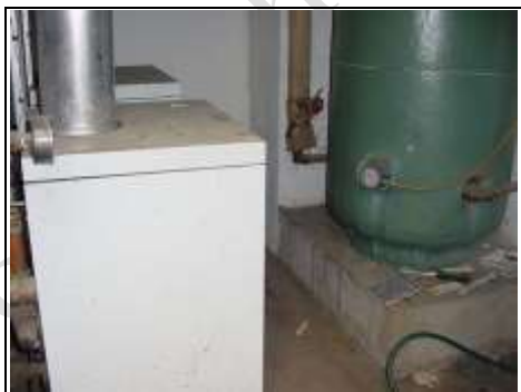
Factory lagged hot water cylinder in middle void
