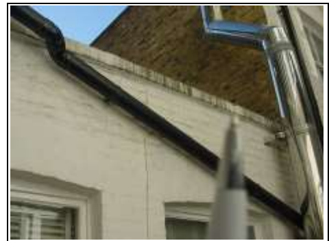
Problem with box gutter over this section which consists of lounge and boiler room
