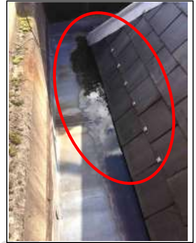
Rear left hand corner – more lead tingles and also ponding within the box gutter
