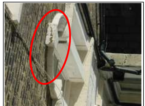
Dampness to the mouldings around the window and the keystone where there is a ledge
