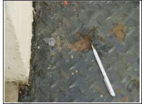
Close up of rusting stairs
