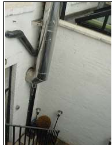
Vent/flue coming from boiler room
