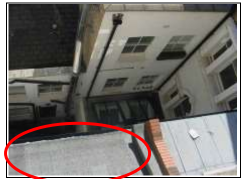
Your patched mineral felt roof to left hand side is in poor condition compared with next door's lead finished roof to the right
