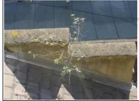
Rear parapet wall/balustrade without box gutter detail. Plants growing from it indicate that dampness is getting in to it
