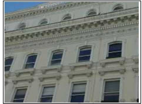
Render to front of property where hairline cracks can lead to dampness coming in
