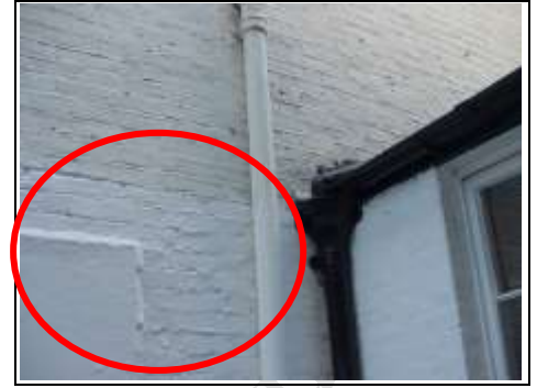
Wall only painted to bottom half
