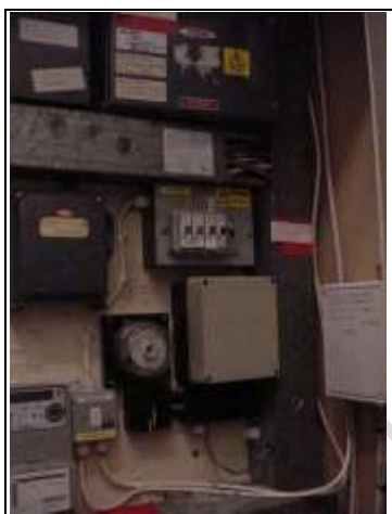
Electrics in cupboard on ground floor
