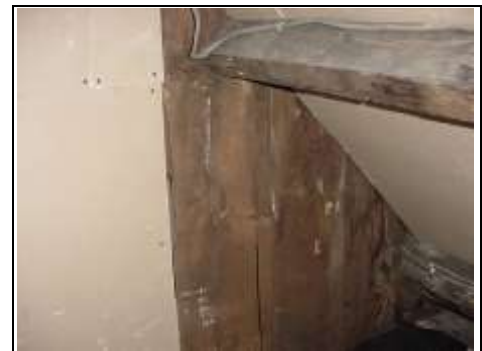
Small bit of roof we could see to the left hand side
