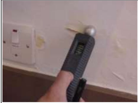
Damp meter readings indicate dampness is coming into the fourth floor via the front parapet wall
