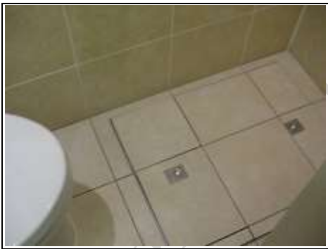
Manhole in lower ground floor apartment
