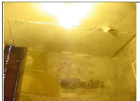
Damp in ceiling to store room off kitchen
