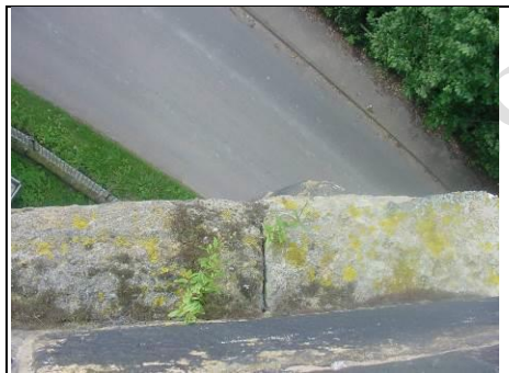
Ledge joints need repointing and growth of vegetation
