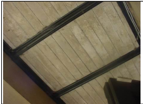
Some of the barrel ceilings / waggon roof are in poor condition
