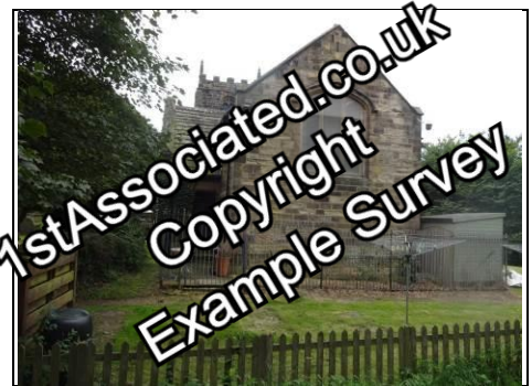
Perpendicular stained glass window externally covered with plastic
