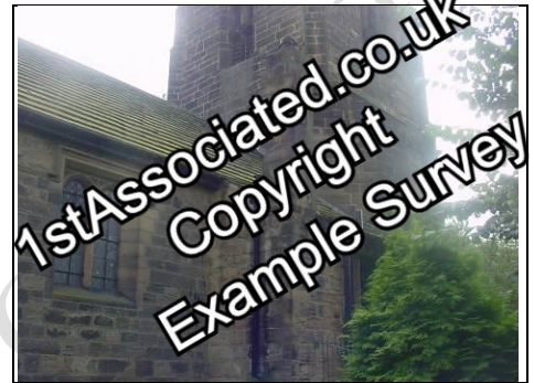
Hopper head and gutters discharge down wall
