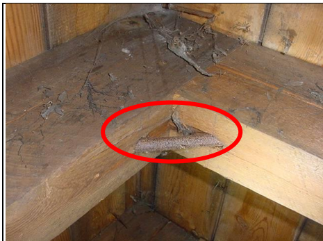
Rusting metal tie bar
