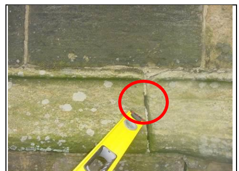
Weathering to pointing
