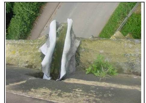
Tower rainwater head that discharges rainwater down the building
