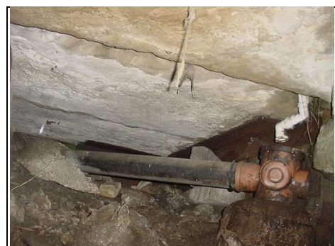
Sump pump or gas supply under the stones
