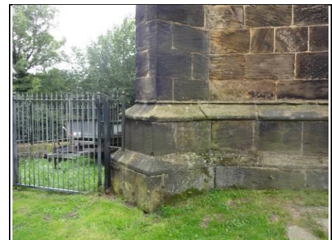
Water runs to the base where there is worn out pointing and deterioration to stonework
