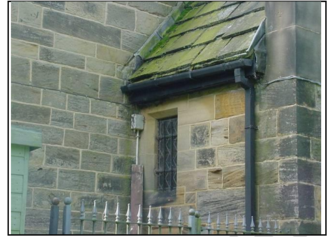
Damaged stonework to north side
