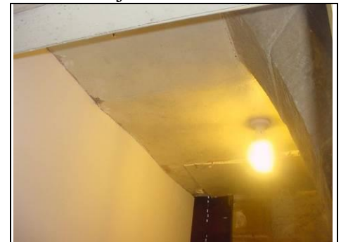
Staining to store room roof
