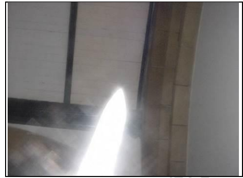
Dampness visible within chancel apartment area
