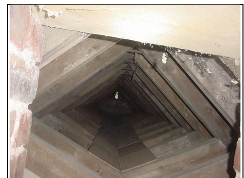
Last bit of roof over Chancel inspected by torchlight only, limited our view
