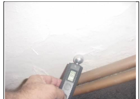
Testing for rising damp
