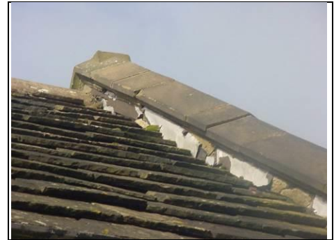
Deteriorating flashing on parapet
