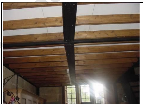
Underside of first floor, see how the steel beam twists with the timbers in it
