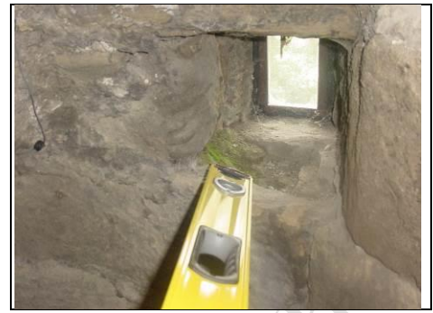
Dampness and moss coming through window
