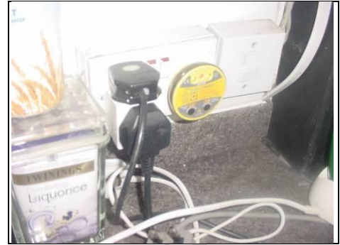
Failed earth test
