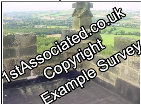
Problems with flashing on roof
