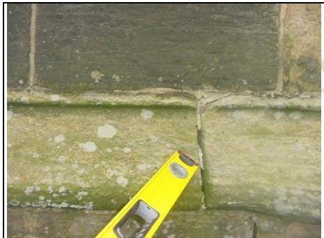
Weathering to stonework and deteriorating pointing
