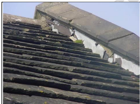
Flashband flashing deteriorating on chancel roof
