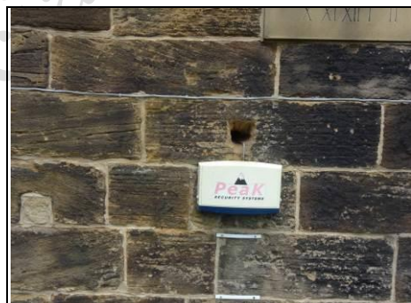
Repairs to stonework generally to south face (and access hole for wasps!) Aerial view – 360 photo
