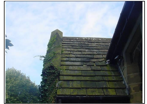
Damaged stone slabs to roof
