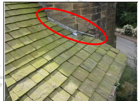
Flashing coming away around Tower
