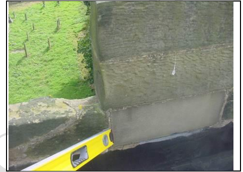
Old repairs to parapet visible
