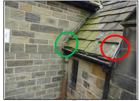
Extra lead added (red oval) and missing lead (green oval). Leadwork needed Aerial view – 360 photo
