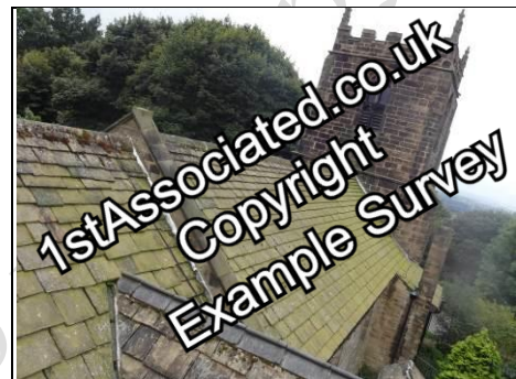
Parapet walls are allowing dampness in Aerial view – 360 photo
