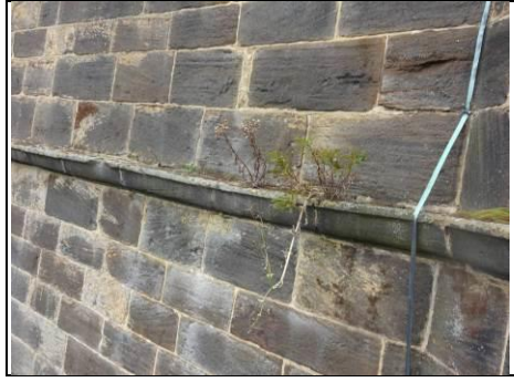
Vegetation growing on wall ledges Aerial view – 360 photo
