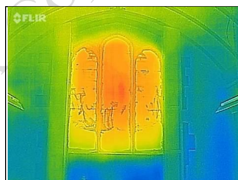
Thermal imaging photo showing heat loss through the window
