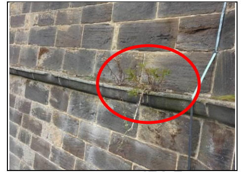
Plants growing out of the ledge Aerial view – 360 photo
