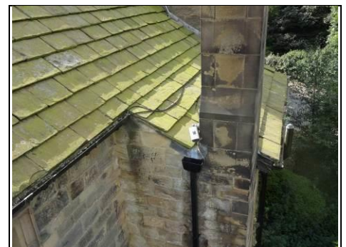
Base of chimney, with overflowing hopperhead to the side.
