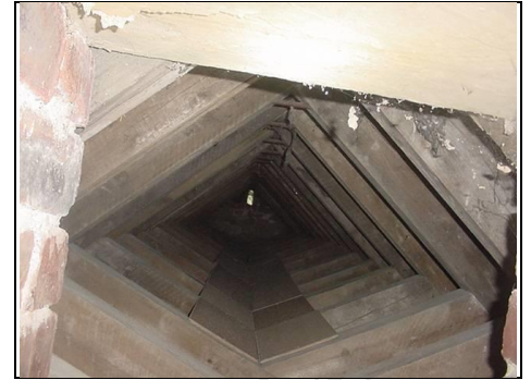
Last bit of roof over Chancel inspected by torchlight only, limited our view
