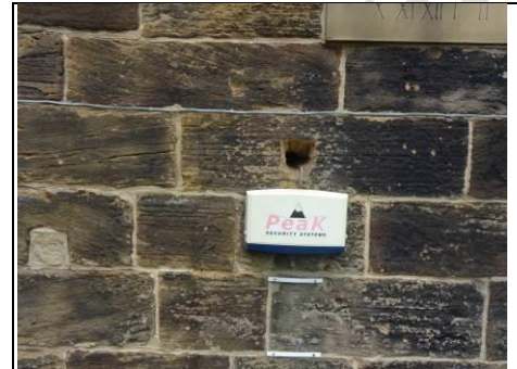
Alarm box on church tower with entrance for wasps just above! Aerial view – 360 photo
