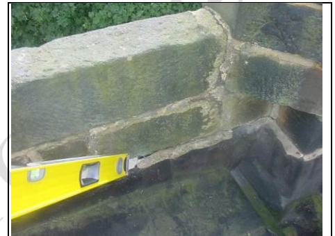
Pointing coming away from the flashing
