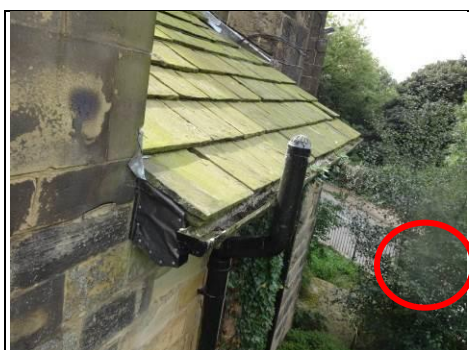
DIY plastic repair to fascia board
