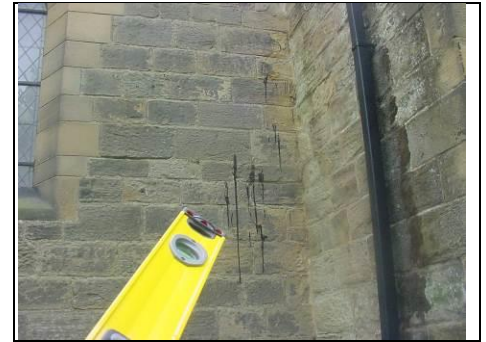
Tar on stonework to rear and downpipe leaking down wall
