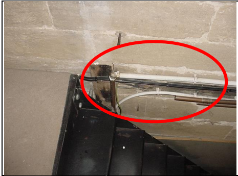
Pipes cut off at top of metal staircase to first floor
