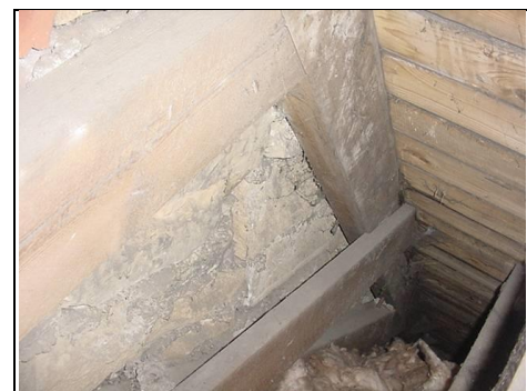
Wall between the Nave and Chancel with brick to the top and stone down the side
