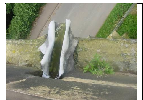
Rainwater gully discharges rainwater down wall
