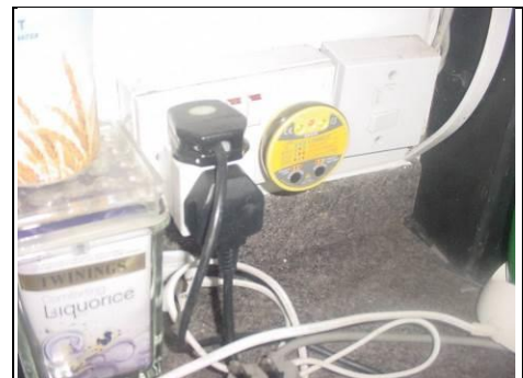
Earth test failed
