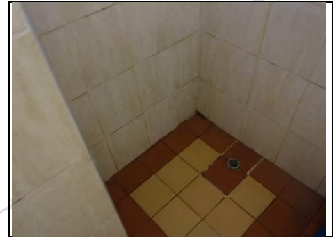
Black mould to tiles in shower room
