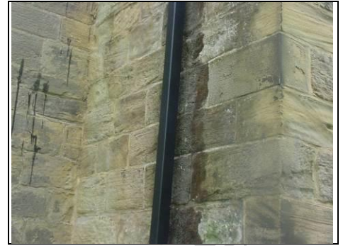
Water discharging down rear left wall next to chimney
