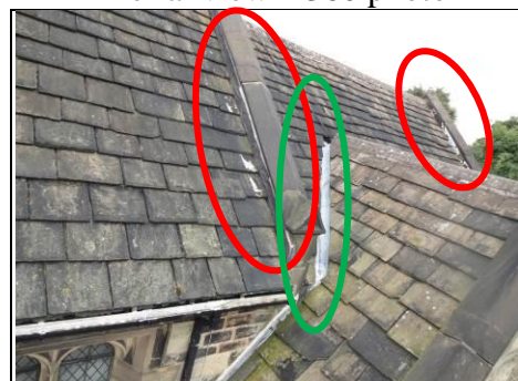
Two main parapet walls with Flashband repairs (red ovals) and valley gutter (green oval)
