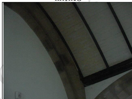
Difference in colour on barrel roof believed to be due to dampness in this area
