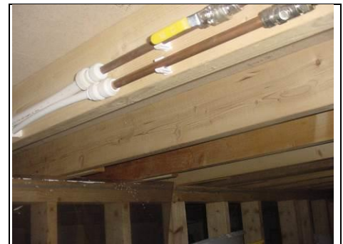
Mix of plastic and copper pipes under the lounge
