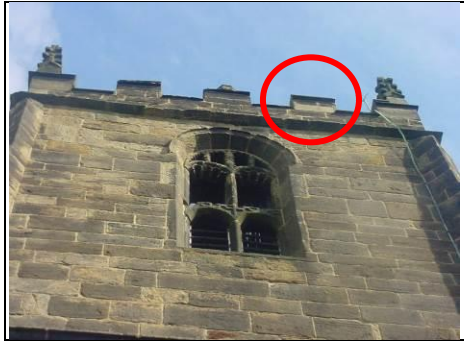
Old repairs to parapet visible
