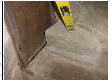
Stone steps to west side of Tower, level indicating new bit of stone added, meaning the door can no longer open
