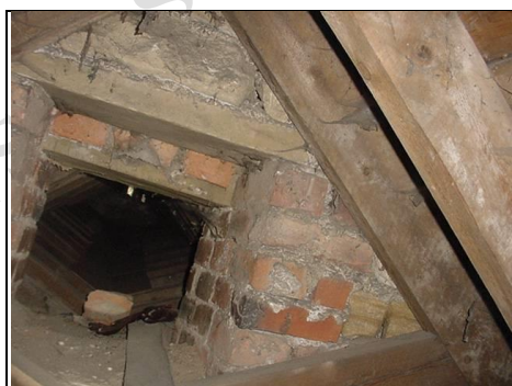
Over Chancel Arch where there is a mixture of brick and stone
