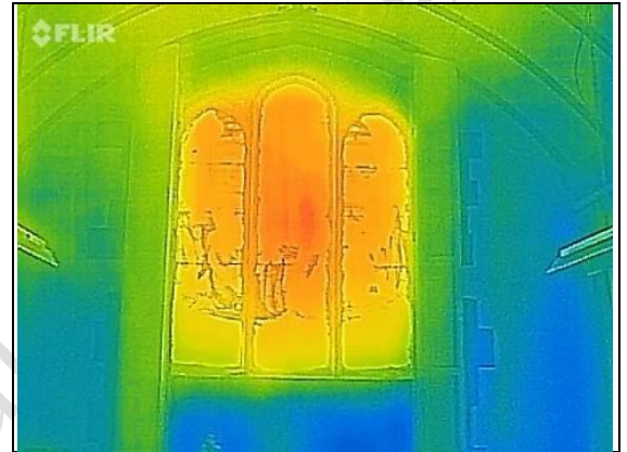
Heat loss through window
