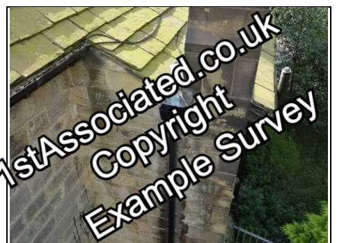
Close up leaking hopper head and gutters, discharging down the wall Aerial view – 360 photo
