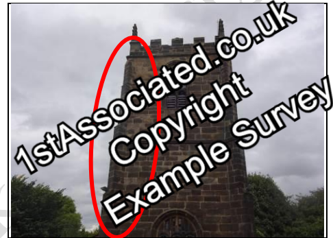
Water discharges down Tower
