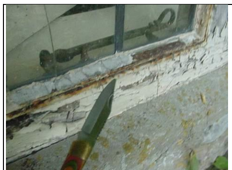
Rusting metal casement window
