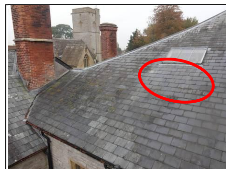
Repairs to slates below roof window Aerial view – 360 photo
