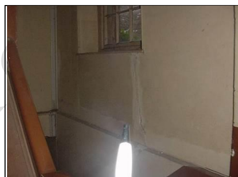
Crack in the wall next to the staff accommodation stairs
