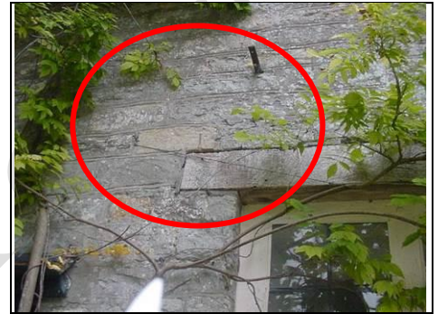
Stonework looks to have been wrongly repointed in cement mortar
