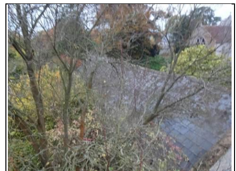
Trees hiding deteriorating rear of stables
