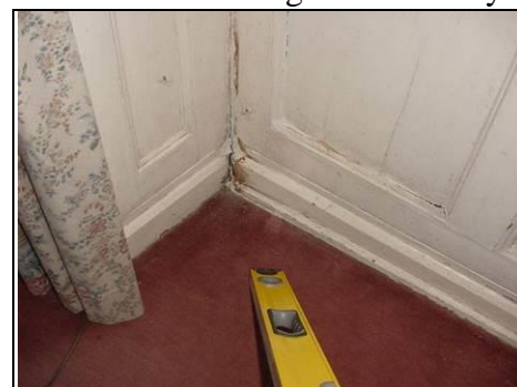
Area where the floor is softer and had a duller thud
