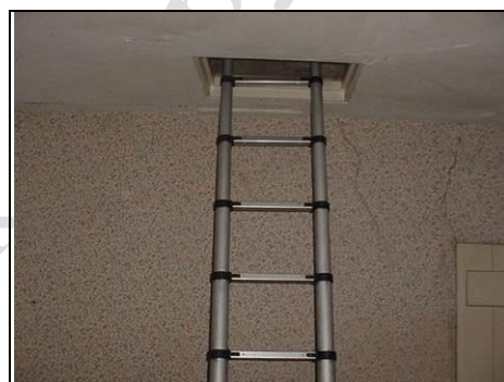
Loft access from staff quarters in the rear roof. Note the cracking to the wall behind the ladder
