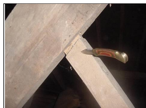
Signs of movement as the tenant joint is coming out
