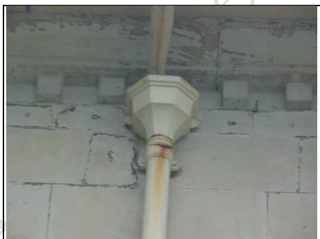
Cracked collar to hopper head and rusting downpipes
