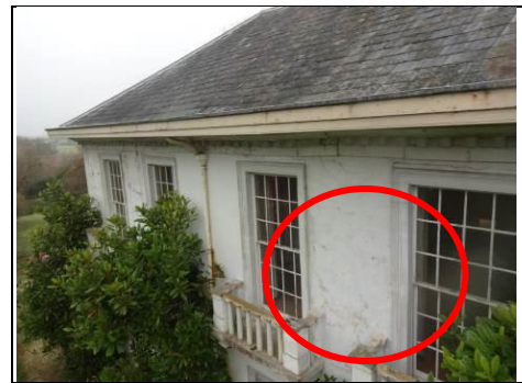
Cracking in wall
