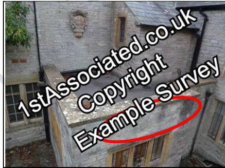
Small flat roof over rear kitchen with pattern staining beneath Aerial view – 360 photo
