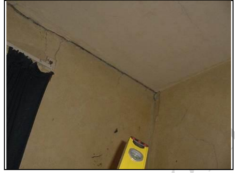
Right wall coming away from inner wall in the utility area
