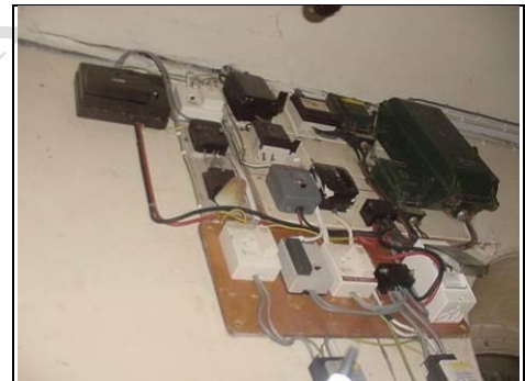
Fuse Board next to staff accommodation staircase
