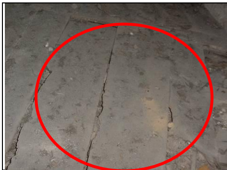
Frass in floor boarding
