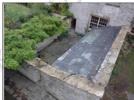
Flashing coming away on pitched slate roof
