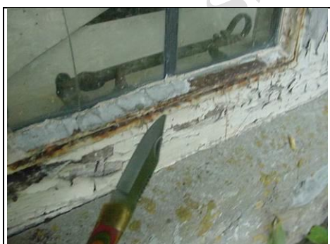
Deteriorating timber window with metal frame
