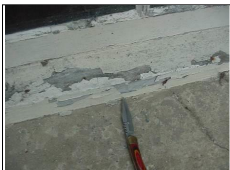
Typical window with flaking paint and bare timber visible
