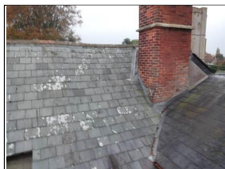
Spalling brickwork Aerial view – 360 photo
