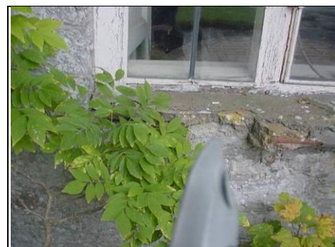
Window sill repaired in cement on right side of property
