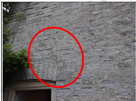
Stepped crack above door Aerial view – 360 photo
