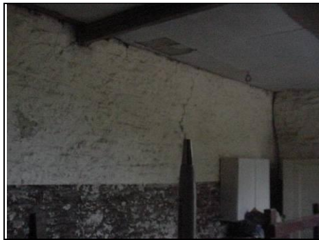
More cracks in garage area
