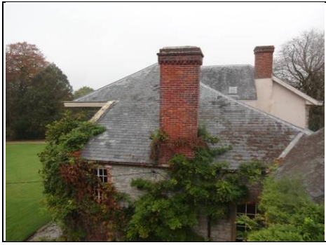
Chimney three to front right side of property (chimney one in background)
