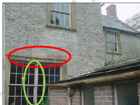
Timber lintel (red oval and window propped up (green oval))
