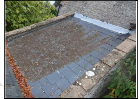
Slates coming away Aerial view – 360 photo
