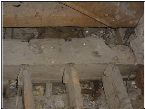
Joint looks to be opening up and repaired, unless this is a style of joint we have not seen before
