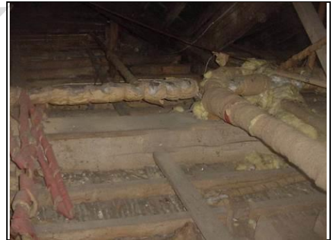
Lagged pipes, may have an element of asbestos
