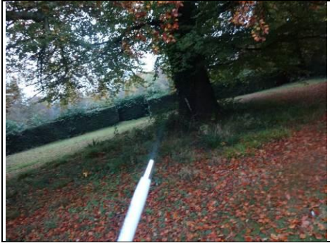
Basic septic tank by tree
