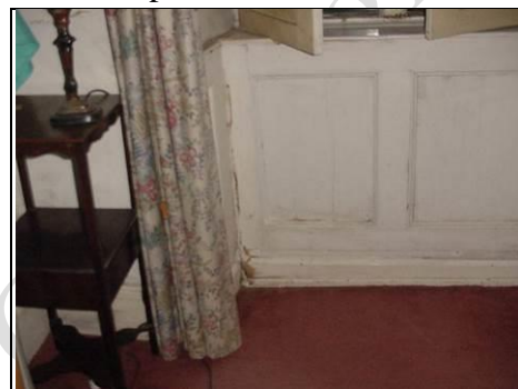
The Room to the front right is where there are signs there is dry
