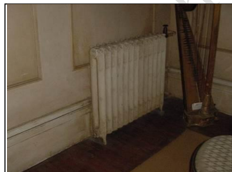
Old school style radiator
