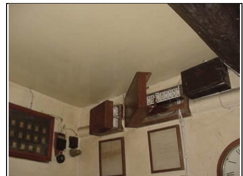
Fuse Board in kitchen area
