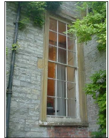
Prop on casement window where there is movement above
