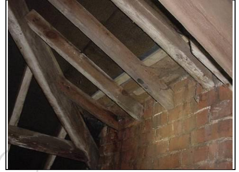
Dampness coming in around chimney one
