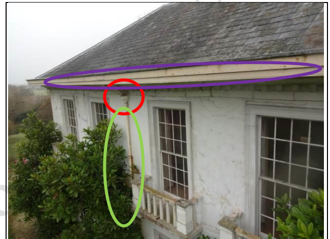
Hopper heads (red), downpipes (green) and wide eave fascias and soffits (purple)
