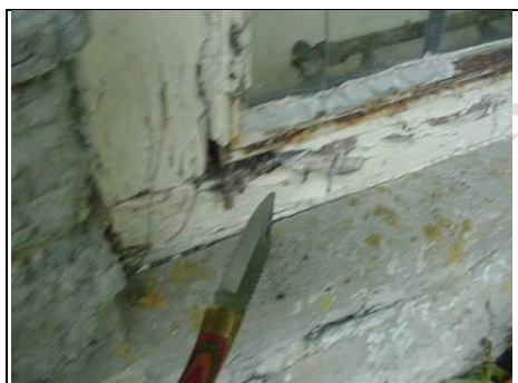
Deterioration to timber
