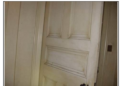
Stained timber door
