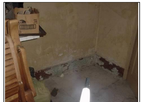
Dampness in the workshop/ old kitchen
