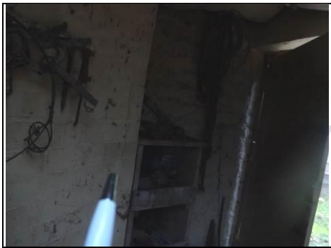
Cracking in tool shed
