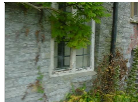
This window on right side of property is in terrible condition
