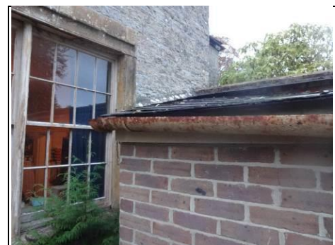
Rusting guttering Aerial view – 360 photo
