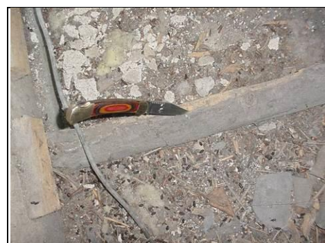
Signs of woodworm to the older timbers
