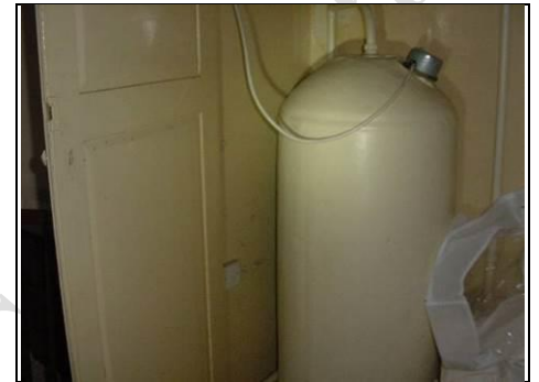
Water tank in left middle room
