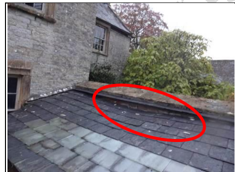
Roof dipping and flashing coming away Aerial view – 360 photo
