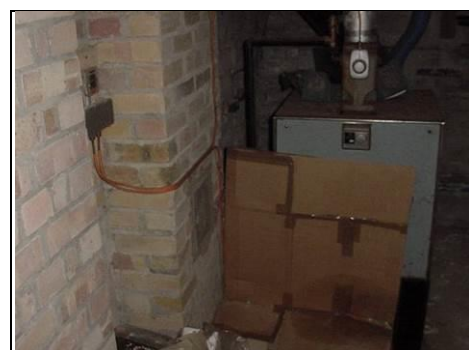
Old boiler in Tank Room
