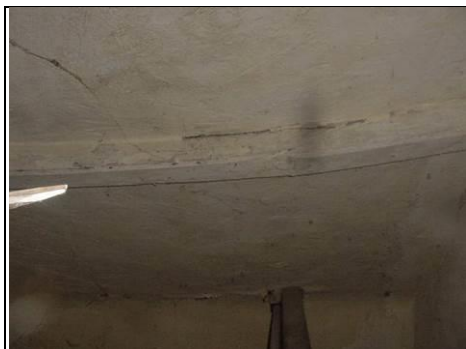
Deflection to purlin
