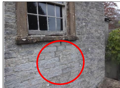
Crack under window on right side Aerial view – 360 photo
