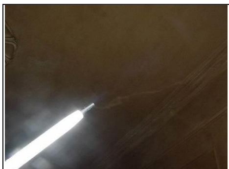
Crack to ceiling in rear left dining room
