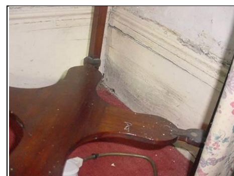
Signs of dry rot
