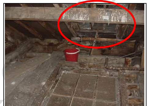
Roof window is leaking. A bucket is never a good thing!
