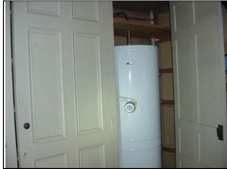
Unvented boiler in linen cupboard
