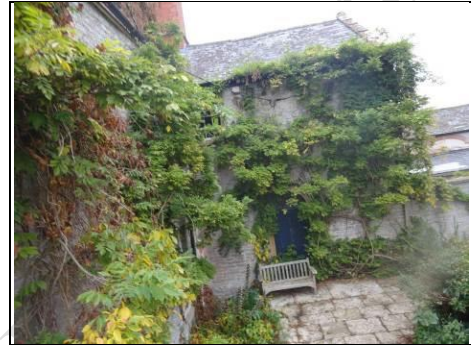
Close up of right side where the wisteria needs cutting back
