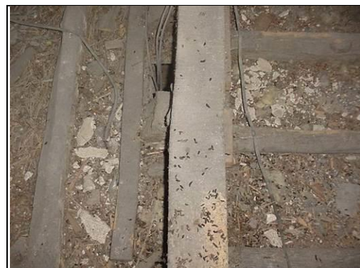
Signs of vermin in the roof
