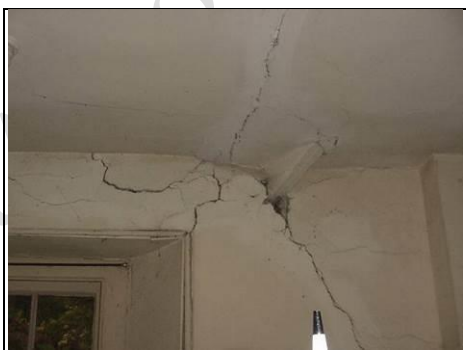
High level cracking to walls and ceiling around window on staircase to staff accommodation
