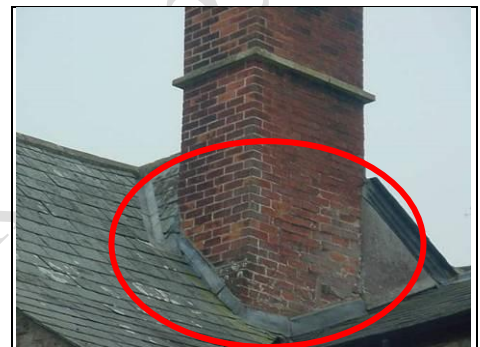
Flashing not cut into the brickwork coursing and weathered brickwork to chimney four
