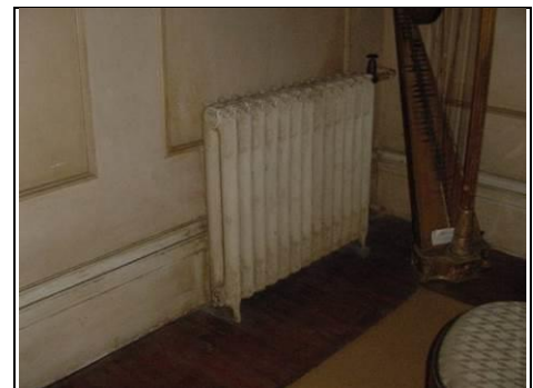
School style radiator
