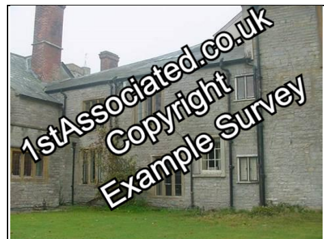
Soil and vent pipe to rear
