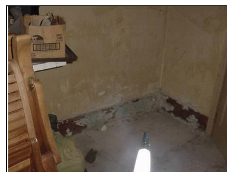
Dampness in the workshop/ old kitchen
