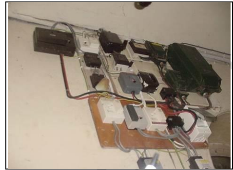
The electrics near to the Right Room
