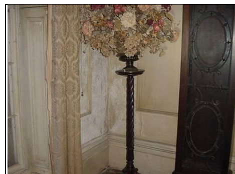
Visible dampness in the formal Drawing Room to front middle
