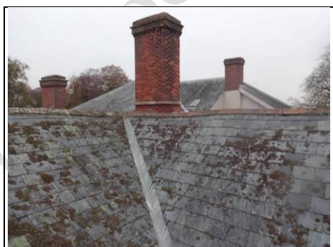
Chimney four deteriorating Aerial view – 360 photo
