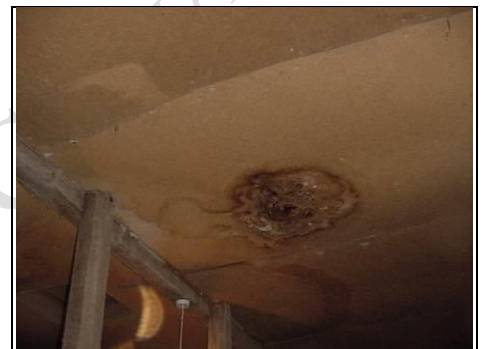
Roof of stable area leaking
