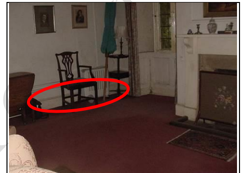
Signs of dry rot in the skirting boards
