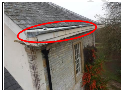
Lead detailing / box gutter on the wide eave fascias and soffits to rear left side Aerial view – 360 photo
