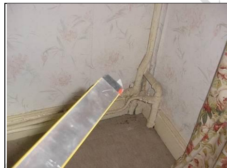
Close up lead pipes
