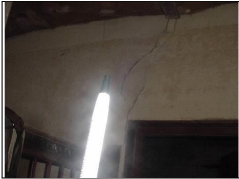
Cracking internally in stables
