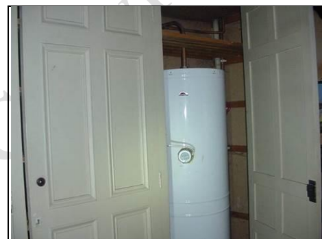
Unvented hot water cylinder in Linen Room
