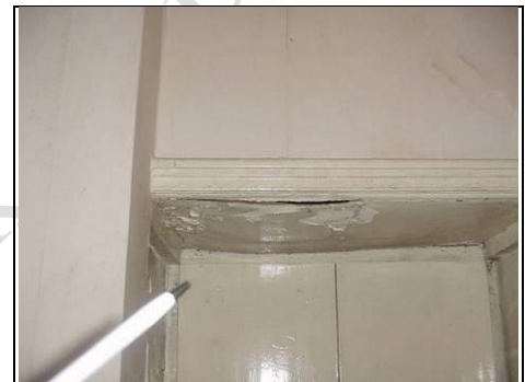
Water damage in cloakroom
