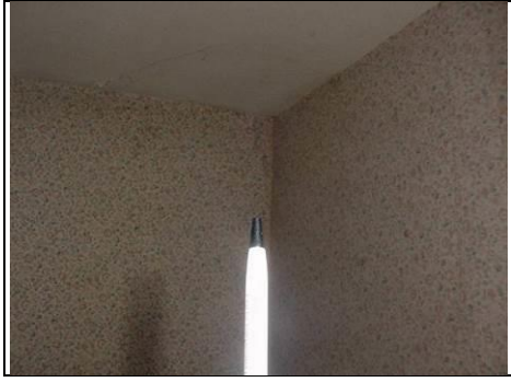
Right wall coming away from main building in the staff accommodation rear bedroom
