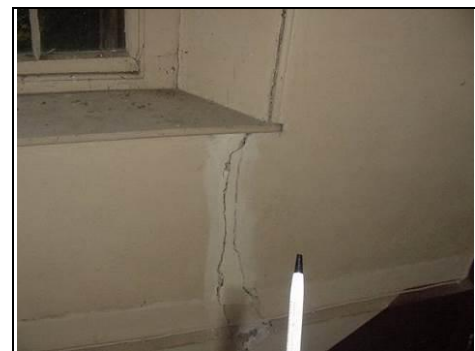
Low level cracking in rear bedroom in staff accommodation
