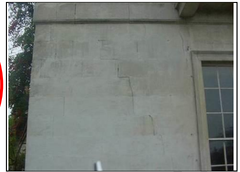
Stepped crack to rear left side at low level
