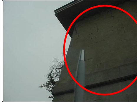
Crack to rear left side at high level
