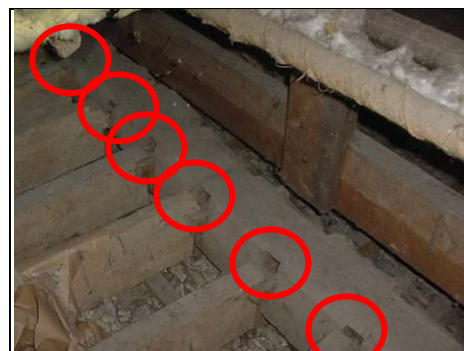
Timber coming out of joints
