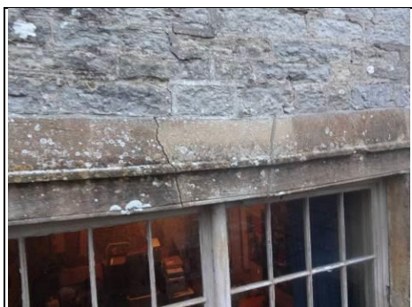
Window is dipping and has a metal prop
