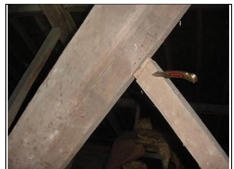
Tenant joint is coming away from the rafter
