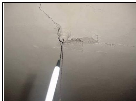
Cracking in ceiling of bathroom
