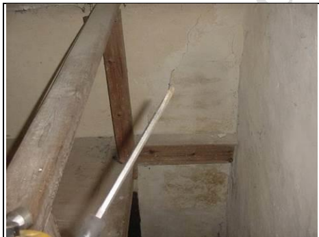
Cracking and dampness coming through walls by rickety staircase to the first floor
