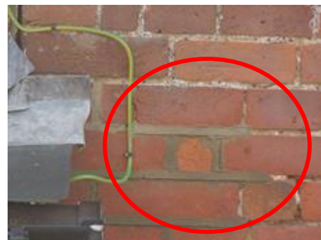
Inappropriate cement mortar will cause damage to soft red bricks
