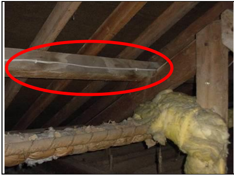
Staining on purlin and possible asbestos
