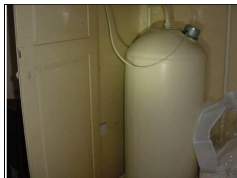
Hot water cylinder in left middle bedroom
