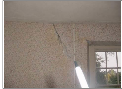
Cracking in staff quarters bedroom
