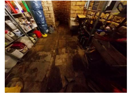
Very wet floor on a dry day
