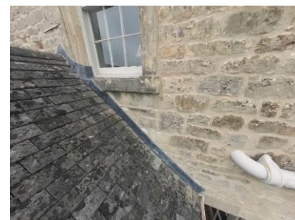
Straight flashing where it meets the wall; prefer a stepped flashing
