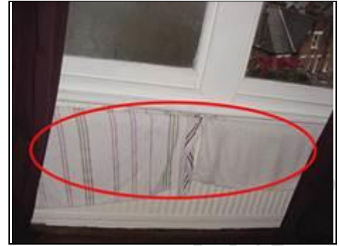
Drying washing on radiators can cause condensation
