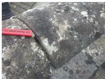
Ridge needs re-bedding
