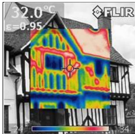
Timber framed House Thermal image showing heat loss
