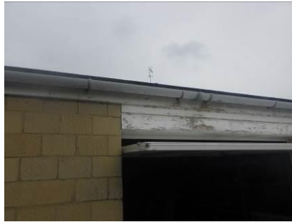
Timber above door needs redecoration
