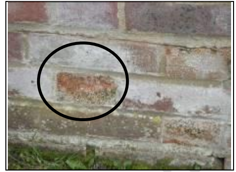
Spalling brickwork and dampness
