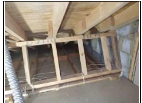
Rear left catslide roof is boarded – no protective underlayer
