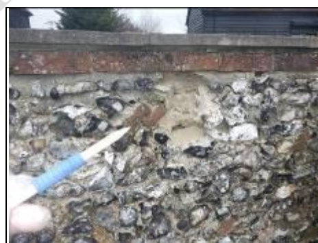
Deteriorating flint wall
