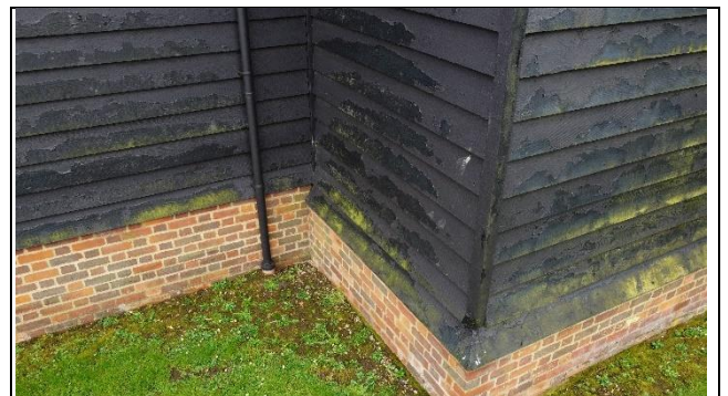
Dampness/moss at low level
