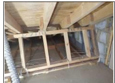
Rear left catslide roof is boarded and supported by purlin with struts at same width as the ceiling joists.
