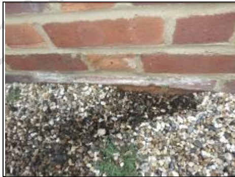
Water sitting against the property due to sloping site
