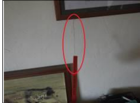
Second vertical crack found on rear wall of ground floor left bedroom
