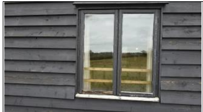
Deteriorating left gable end window ~ Aerial View - 360 Photo ~
