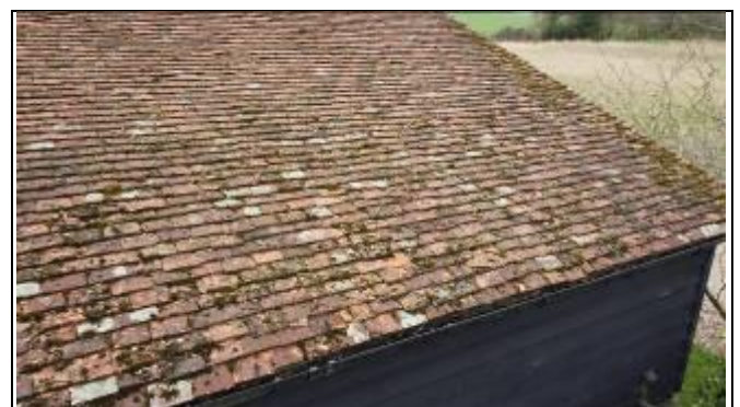
Moss to roof indicating surface starting to deteriorate ~ Aerial View - 360 Photo ~
