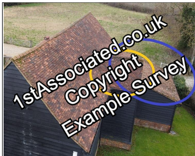
Rear left shallow pitched roof (blue) Stair area (yellow) ~ Aerial View - 360 Photo ~
