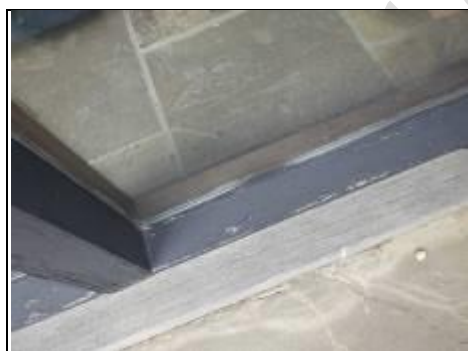
Weathering to timber at base of window within entrance to old barn
