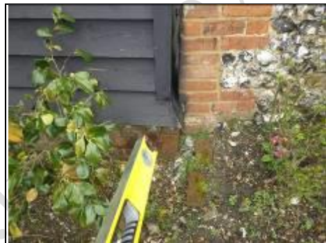
Deterioration to angle timber over brickwork
