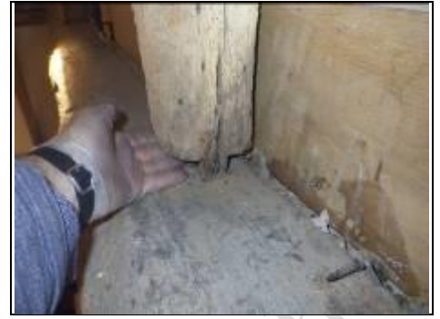
Vertical timbers mortise and tenon joint not working
