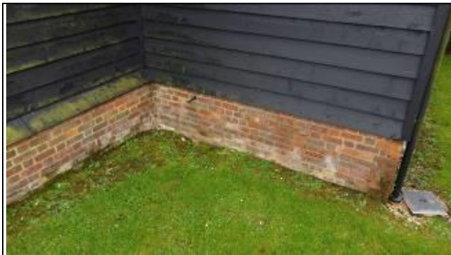
Dampness to rear of property ~ Aerial View - 360 Photo ~
