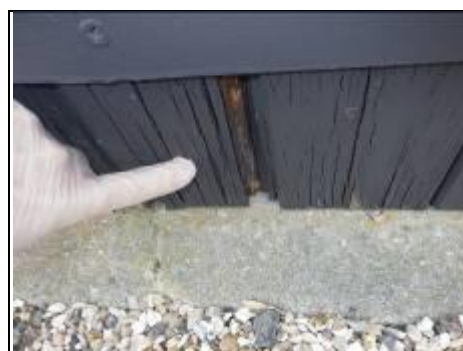
Deterioration to base of ledge and brace doors
