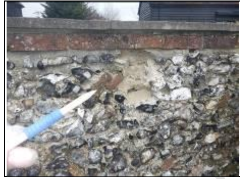
Deteriorating flint wall
