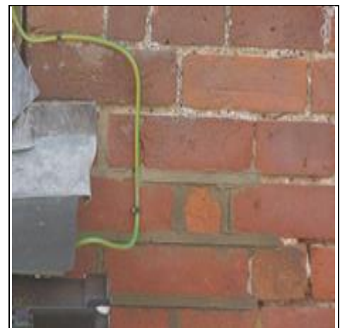
Inappropriate cement mortar will cause damage to soft red bricks
