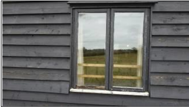
Deteriorating left gable end window ~ Aerial View - 360 Photo ~
