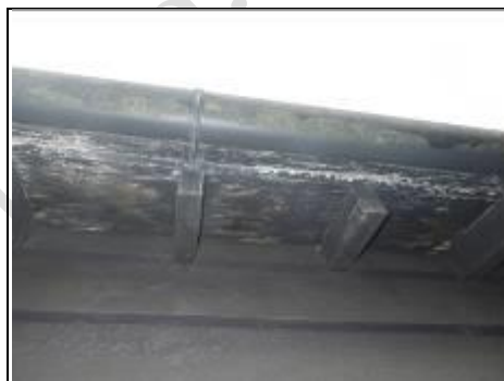
Exposed rafter feet deteriorating
