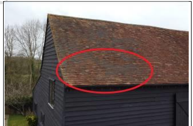
Front left problem area ~ Aerial View - 360 Photo ~
