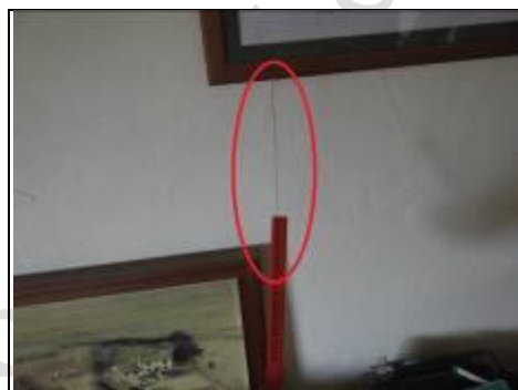
Second vertical crack found on rear wall of ground floor left bedroom
