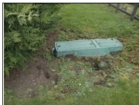
Water treatment system
