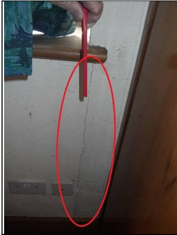
Vertical crack in ground floor left bedroom
