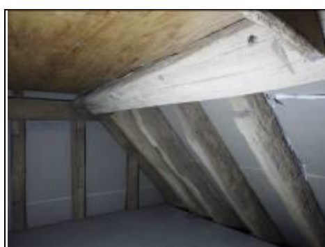
Limited access to right Timber plywood boarding above the collar area
