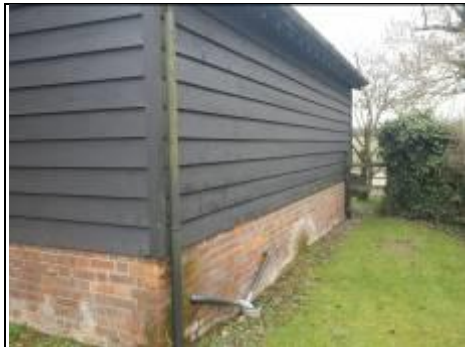
Dampness to rear of the cat slide roof/left bedroom
