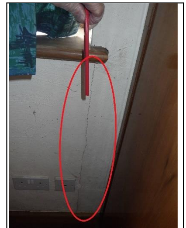
Vertical crack in ground floor left bedroom
