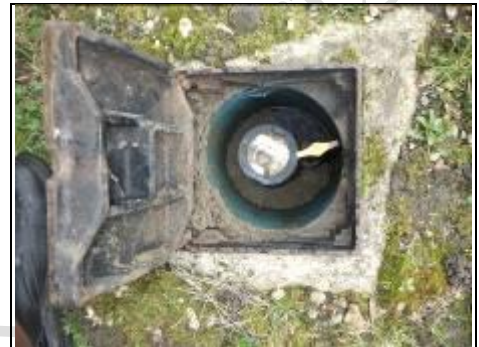
External stopcock on right hand side within garden
