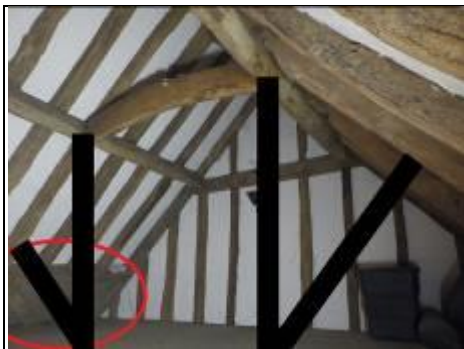
Queen post frame missing to the left side of the property
