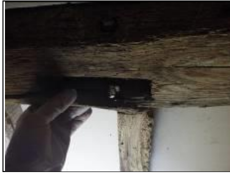
Old fixing points show many alterations to the timber frame
