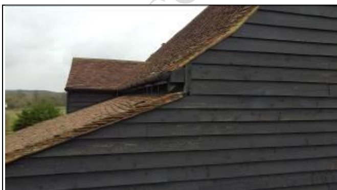
Step in roof from main roof onto cat slide roof ~ Aerial View - 360 Photo ~
