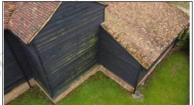
Moss to middle rear weatherboarding externally ~ Aerial View - 360 Photo ~
