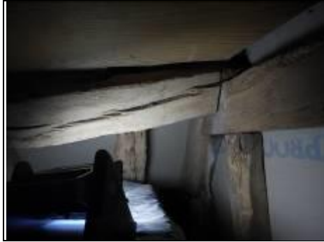
Splits in timber
