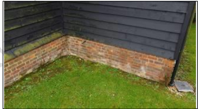
Dampness to rear of property ~ Aerial View - 360 Photo ~
