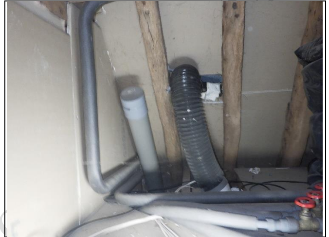
Internal soil and vent pipe and Durgo valve ~ Aerial View - 360 Photo ~
