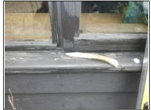
Work required to timber windows
