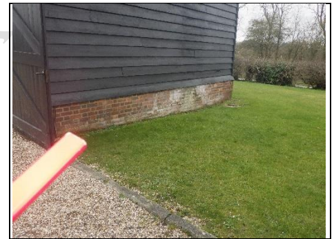
Dampness/deterioration to right gable
