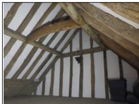
General view of left area where we believe queen post truss would have originally been
