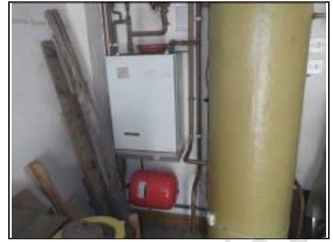
Hot water cylinder
