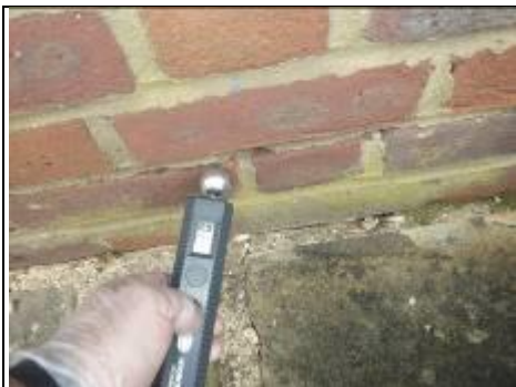
Dampness/moss visible to base of the property
