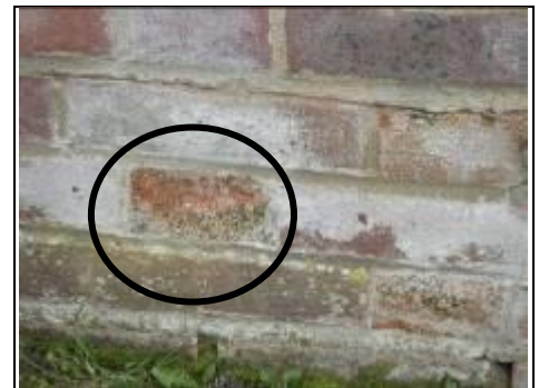
Spalling brickwork and dampness
