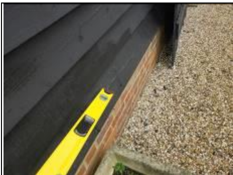
Angle timber over brickwork would this be better in lead this would need conservation officer's approval
