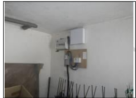
Dated fuse board
