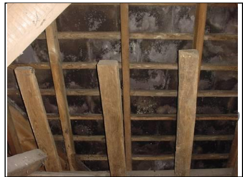
No protective underlayer to older style construction
