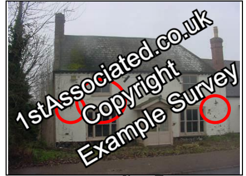
Cracking and tie bars
