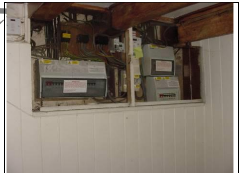
Electrics in the bar area
