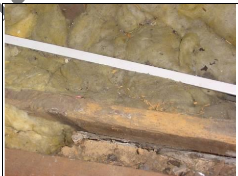
Woodworm in the roof
