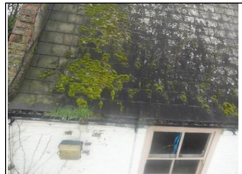
Moss on roof and grass growing in gutter to main roof front left
