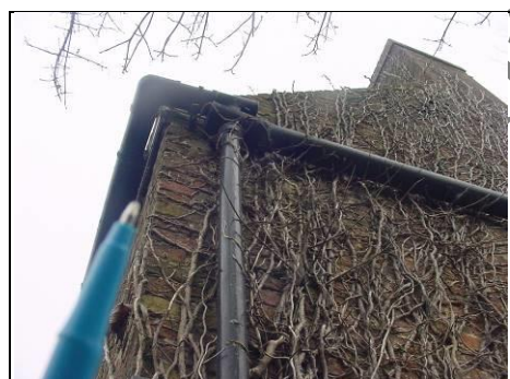
Ivy causing deterioration
