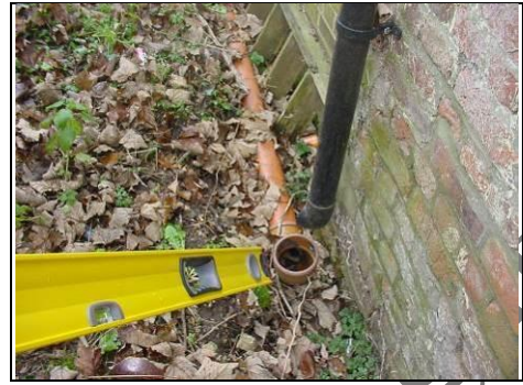
Far left side gutter not joined
