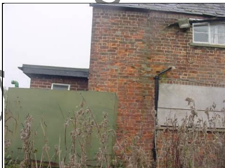
Soil and vent pipe draining away from the bathroom on top floor
