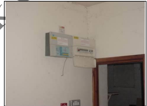
Fuse Board in the function room
