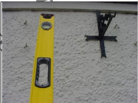
Vertical hair line cracking
