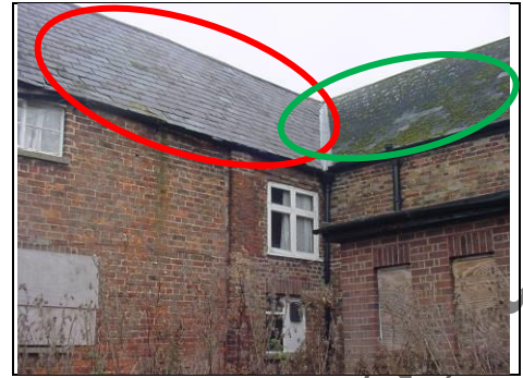
Main rear left roof to rear showing mix of natural slates (red oval) and manmade (with moss on it) (green oval)
