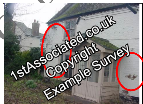
Bricks re-created to left and right in we believe a cement mortar
