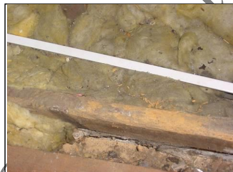
Woodworm in the roof
