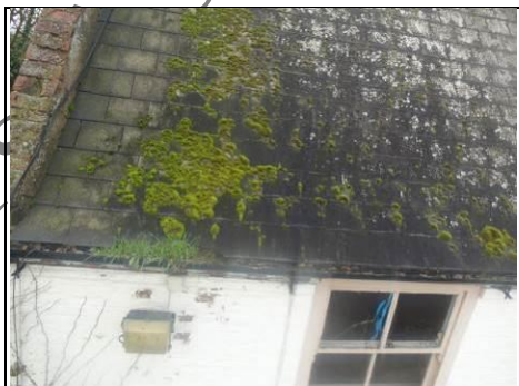
Grass growing in the gutter
