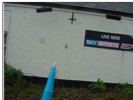
Horizontal cracking and the black area to the base where the drip is
