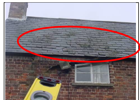
Slipped slates to the rear left
