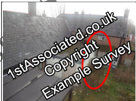
Cracking to the rear right Aerial view – 360 photo
