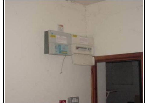
Electrics in the function room
