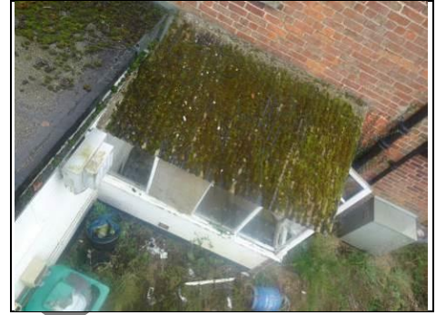
Asbestos roof to the rear entrance
