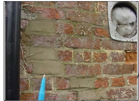
Ad-hoc pointing in cement mortar
