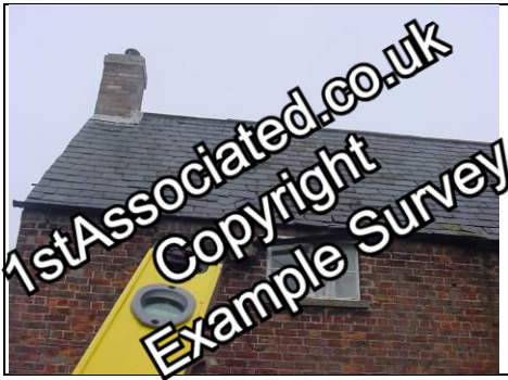
Slipped natural slates to main roof rear left
