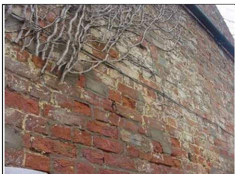
Cement repointing, bricks replaced with cement mortar, lime wash and ivy
