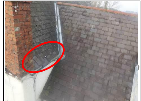
Slipped slates and lead tingles to the front right roof Aerial view – 360 photo
