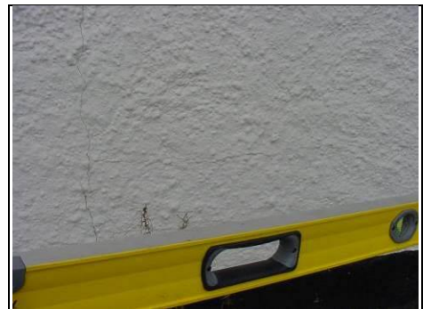
Horizontal hair line cracking
