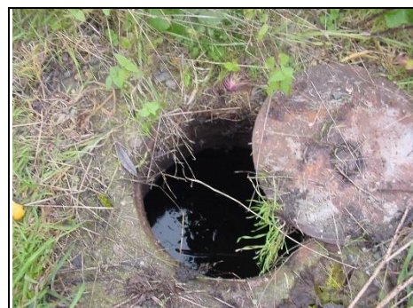
Septic tank / well
