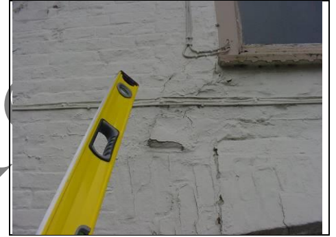
Cracking to the window
