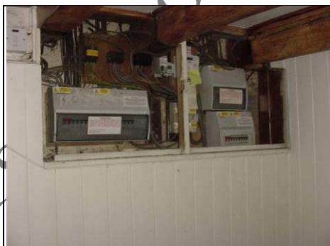
Fuse Board in the bar
