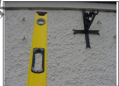
Crack and possible tie bar
