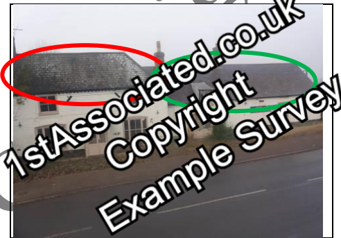
Main roof left (red oval) and right (green oval) Aerial view – 360 photo
