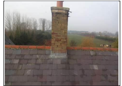
Front right chimney needs re-pointing at the base Aerial view – 360 photo
