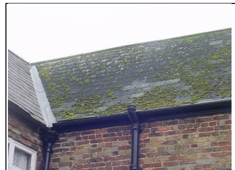
Cast iron soil and vent pipe to rear left
