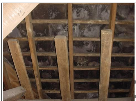
No protective underlayer to the left side of the roof
