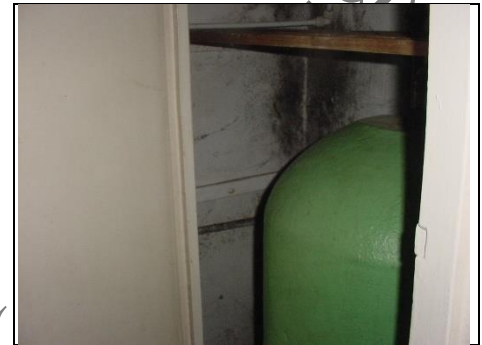
Hot water cylinder
