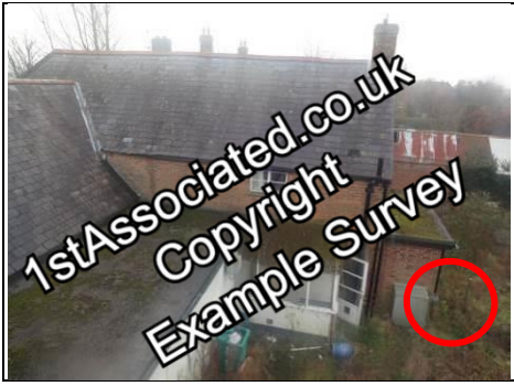
Soil and vent pipe Aerial view – 360 photo
