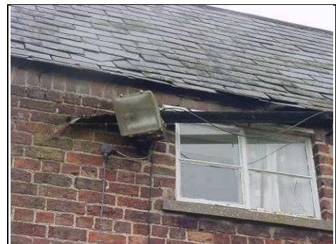
Gutter falling off
