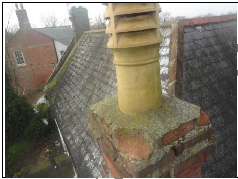
Chimney in below average condition Aerial view -360 photo
