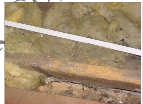
Woodworm in the roof
