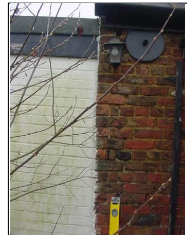
Brickwork with problems to the rear right
