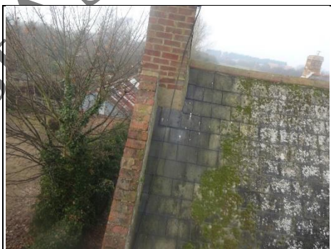
Moss on roof Aerial view -360 photo
