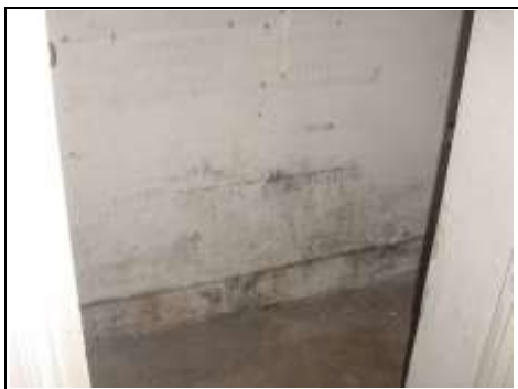
Black mould on wall of cupboard
