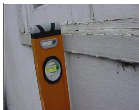
Old Tudor properties often have walls that are out of true or not straight. The level shows just how far the property is leaning. A survey will advise you if this is a problem or not
