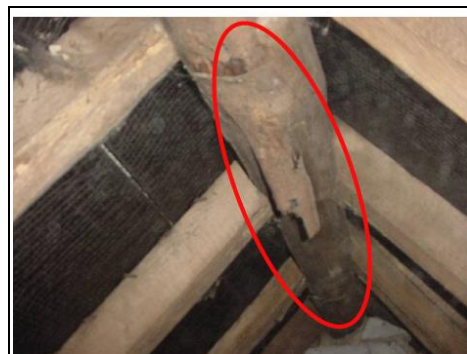
Timber roof structure with ridge timber circled. This is cracking is it important?
