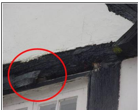
Repairs have been wrongly made to this timber frame in cement or plastic wood instead of splicing with new timber
