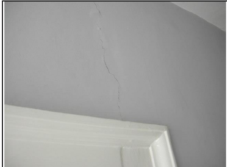
Internal wall cracks
