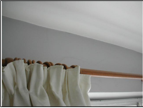
Cracks in external wall above window
