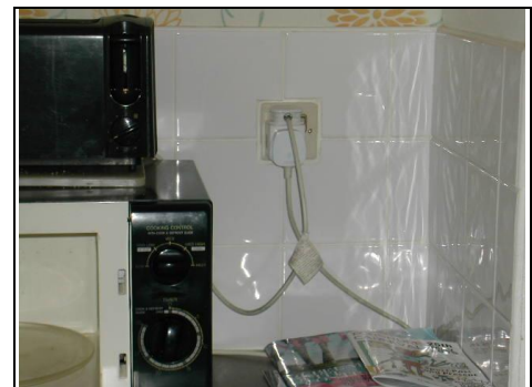
Older style sockets
