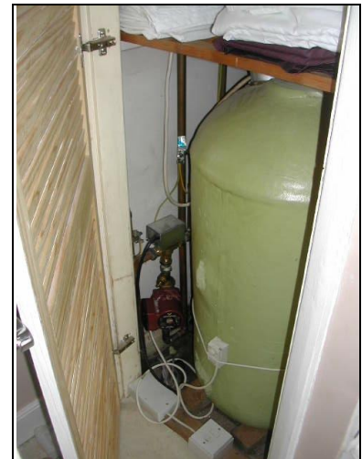
Hot water cylinder
