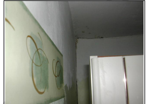
Cracks in Bedroom 3
