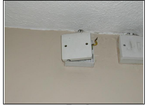
Loose electrical box
