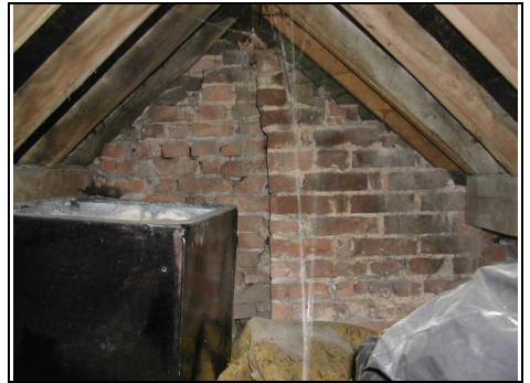
Deflection in end wall
