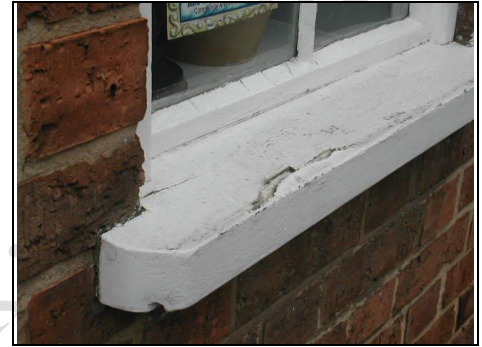
Poor decorative condition
