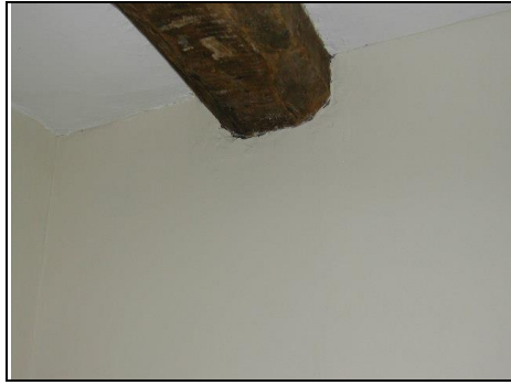
Cracks around centre beam
