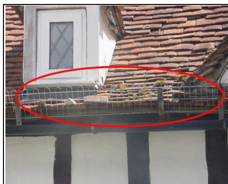
Old peg tiles that are likely to slide off the roof so a slate guard or in this case a tile guard has been used
