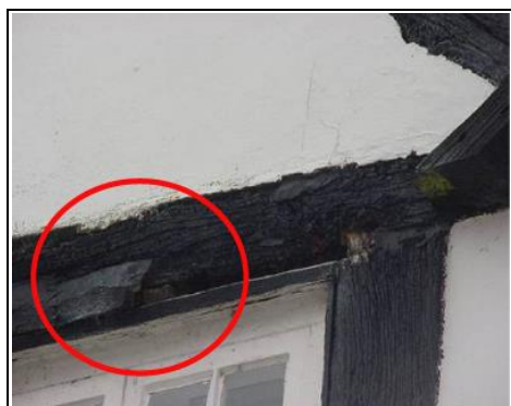
Repairs have been wrongly made to this timber frame in cement or plastic wood instead of splicing with new timber
