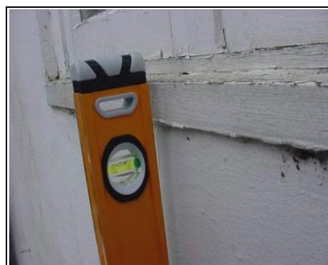
Old Tudor properties often have walls that are out of true or not straight. The level shows just how far the property is leaning. A survey will advise you if this is a problem or not
